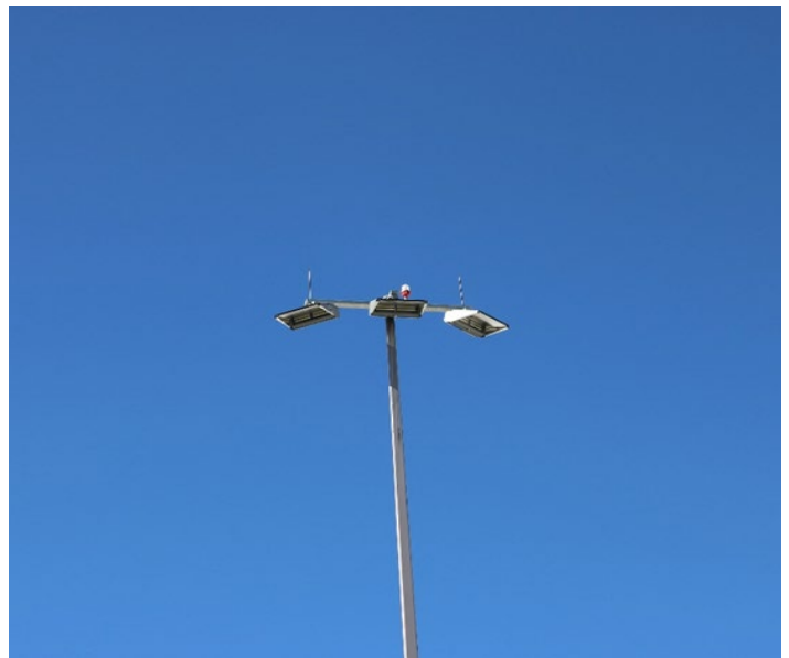
After - (3) 600-watt LED Fixture
