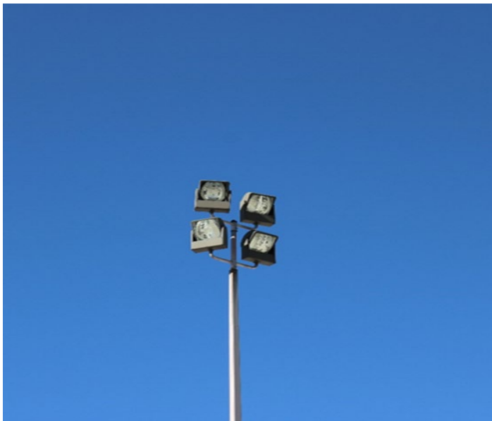
Before - (4) 1,000-watt HID Fixture
