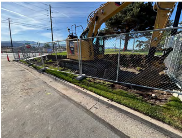
NVE Utilities at Terminal Way
