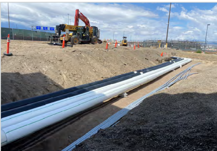
CUP Trench Area 1 Hydronics
