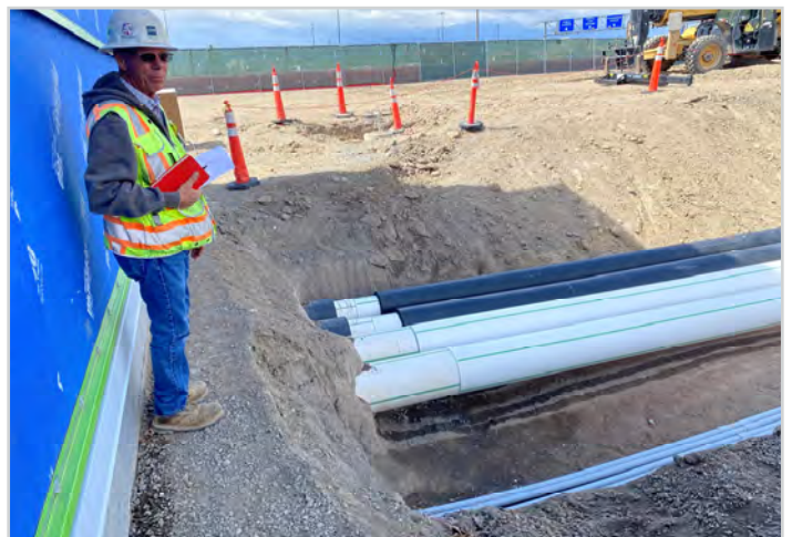
CUP Trench Area 1 Hydronics
