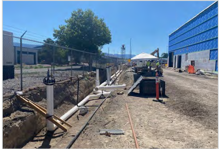
Fluid Cooler Piping
