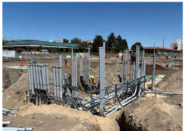
Garage MDF and Electrical Room Utilities
