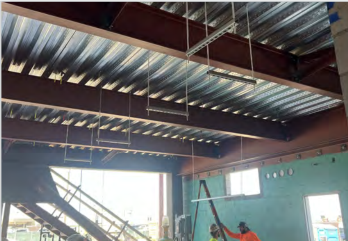
HVAC Ceiling Hangars
