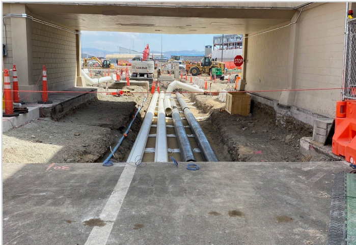
Concourse A - Hydronic Piping
