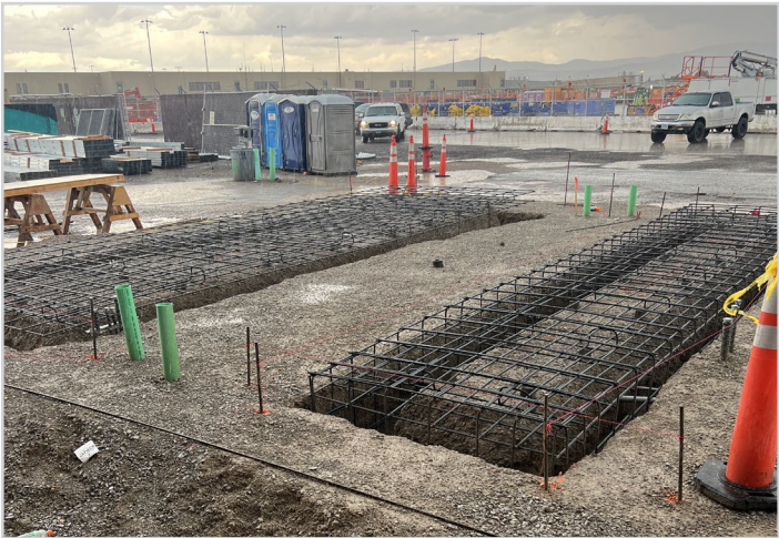
Mechanical Equipment Pads
