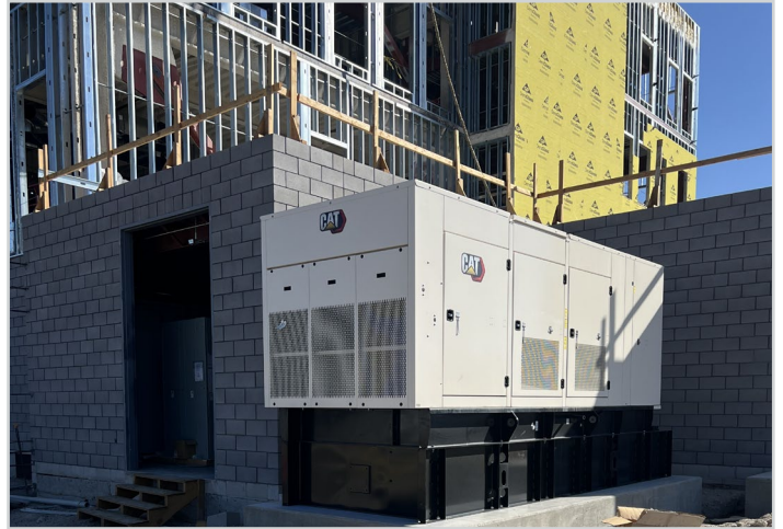
Building Emergency Generator in Place
